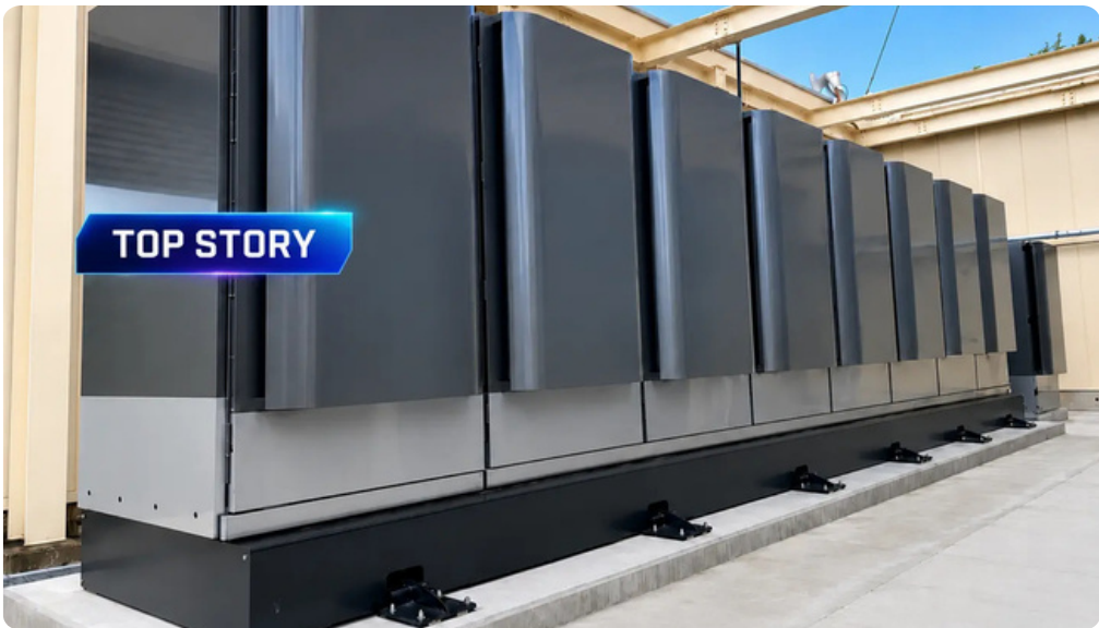
Fuel-cell-based on-site electricity systems
